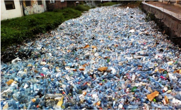
Plate 5.9: PBWS blocking drainage
