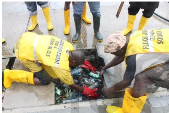
Plate 5.15: PBWS being removed from a blocked drain
