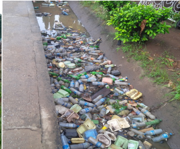
Plate 5.14: PBWS blocking drainage
