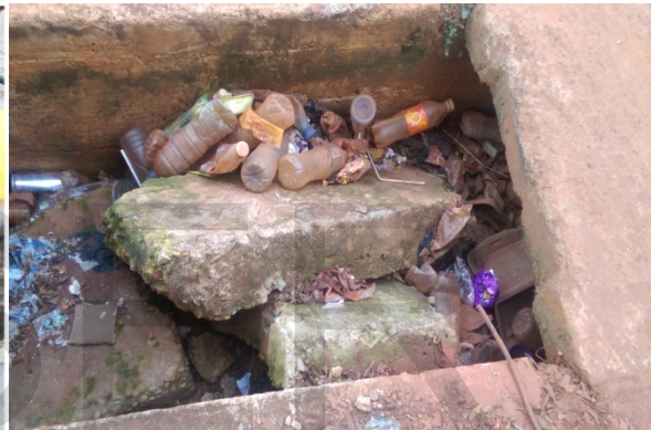
Plate 5.16: PBWS blocking drainage in Enugu
